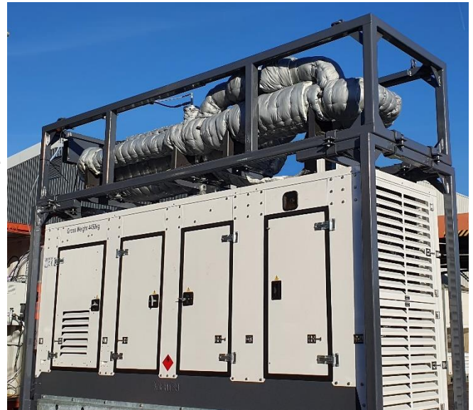
photo: 125 kVA genset met Discom Stage 5 frame
